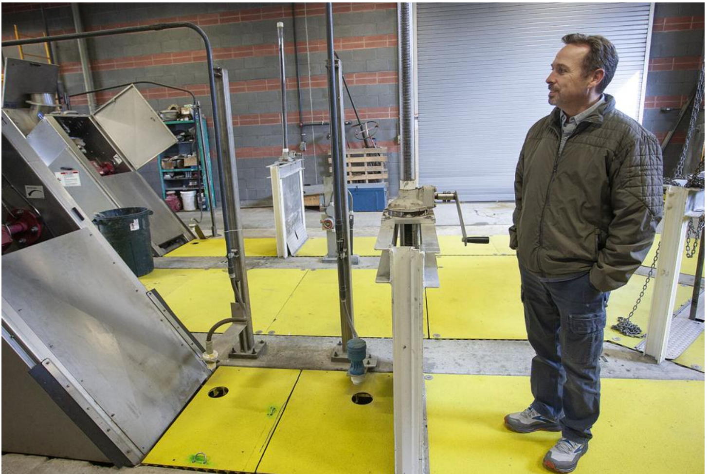
Tony Harmon, superintendent of the Caldwell wastewater treatment plant, talks about the treatment process during a tour of the facility Wednesday.
