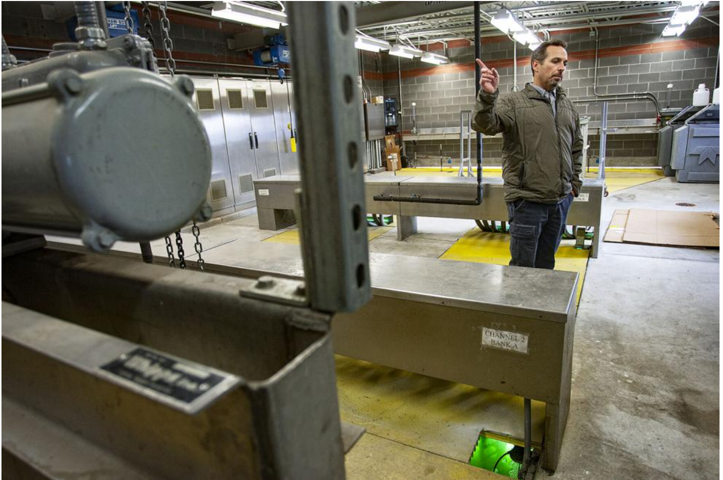
Tony Harmon, superintendent of the Caldwell wastewater treatment plant, talks about the process while standing in a UV treatment area Wednesday.
