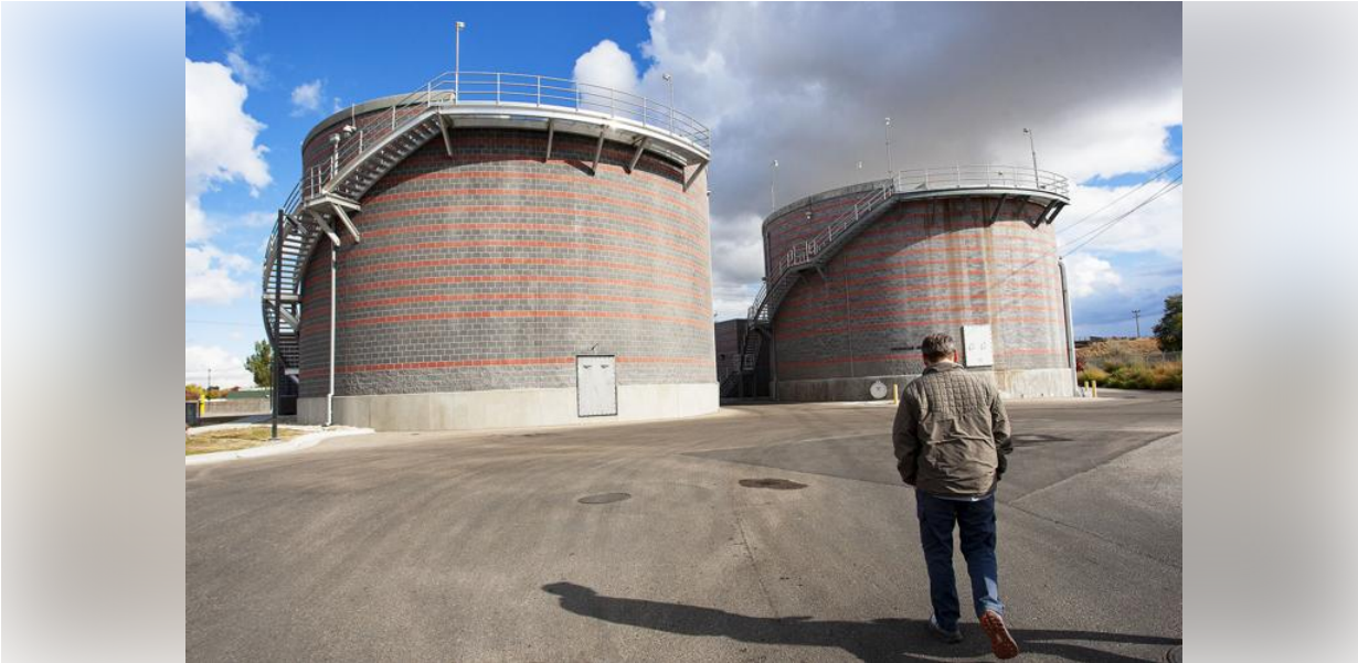
Tony Harmon, superintendent of the Caldwell wastewater treatment plant, walks toward a pair of digester tanks during a tour of the facility Wednesday. The plant has not had any permit violations since a major upgrade in 2019.
